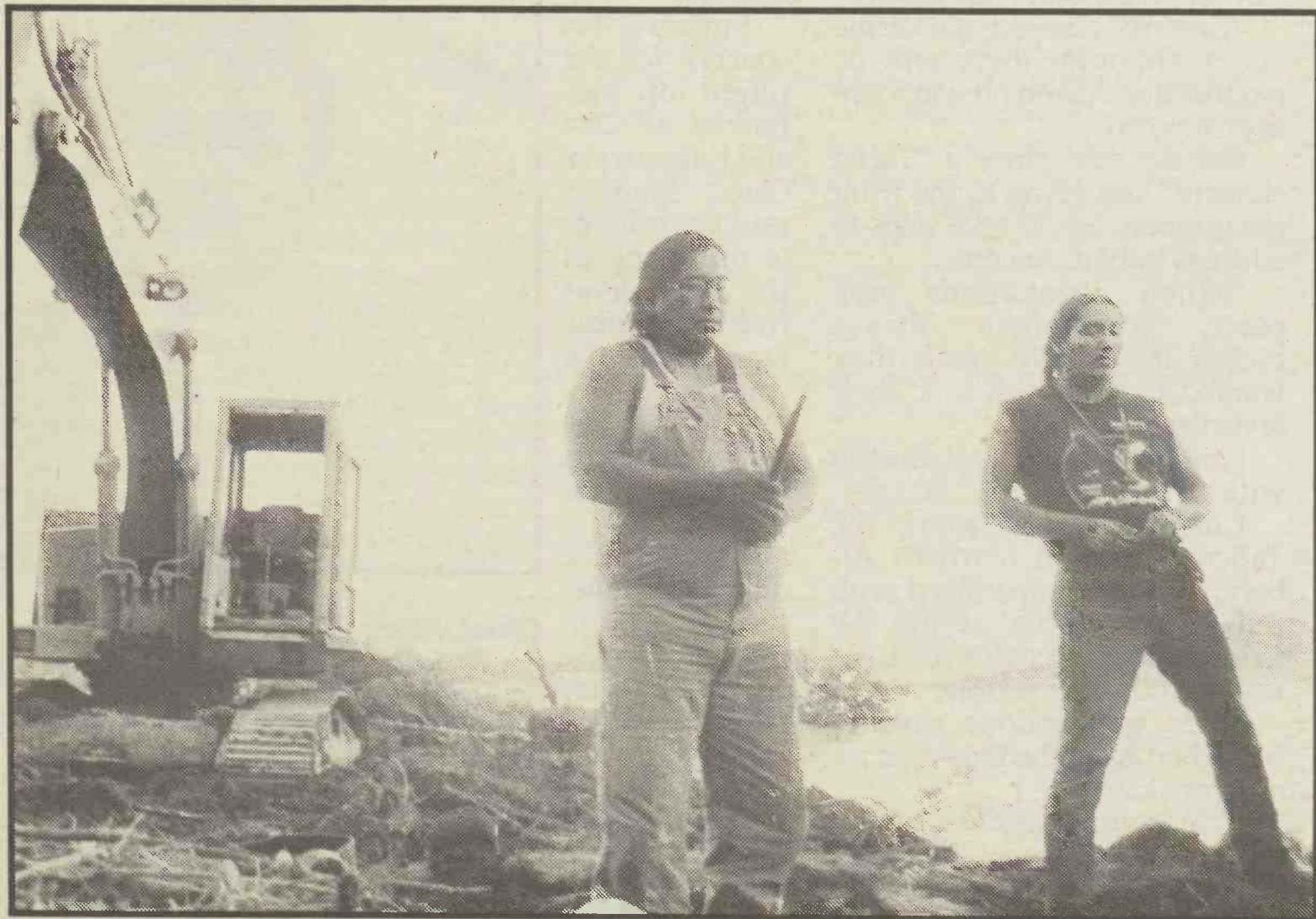
The Lone Fighters Society held a pipe ceremony and made an offering to the river before the final excavation took place.
