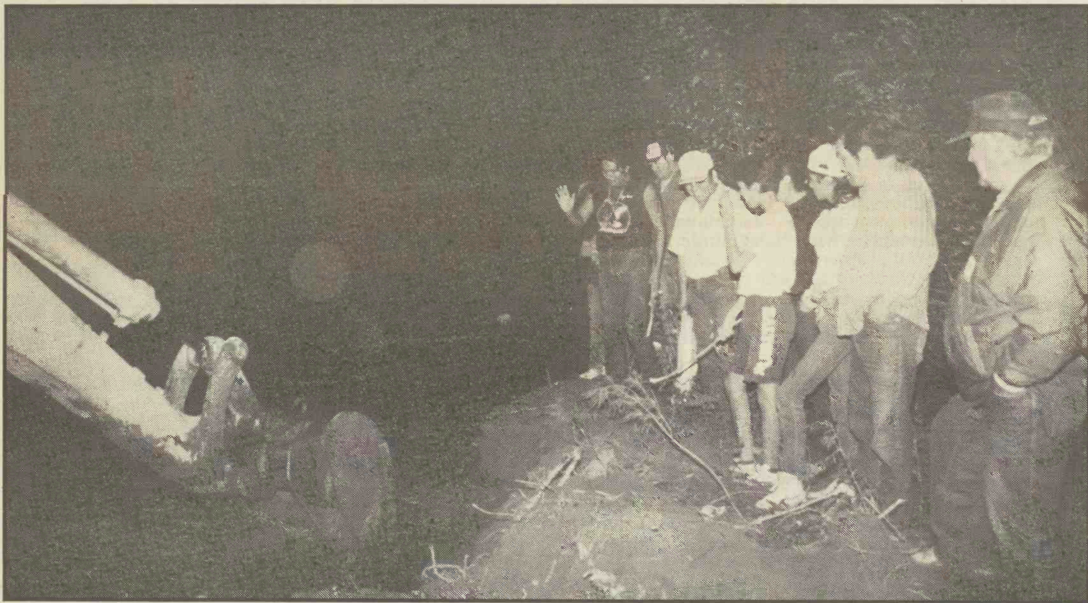
Milton Born With A Tooth directs the excavation of the last few feet before the canal is complete
